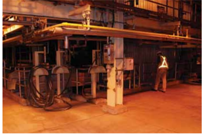
This is the bottom area of the biomass power boiler, where the burning occurs in a totally enclosed system.
